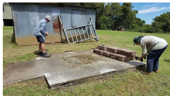
The boys removing bricks and reo from the slab near the helipad
