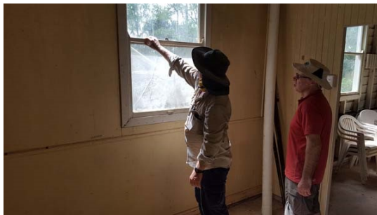
Broken window pane covered with perspex
